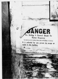
More than two dozen buildings have been declared unsafe by the county—a sign of the neglect that followed in the wake of four killings there 20 years ago.
