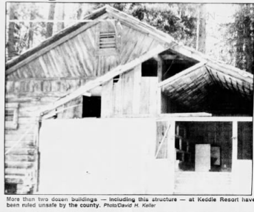
More than two dozen buildings — including this structure — at Keddie Resort have been ruled unsafe by the county. Photo/David H. Keller
