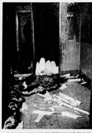
ELEVATOR RUINED BY FIRE ON 2ND FLOOR. Electronics Equipment in Area Destroyed
