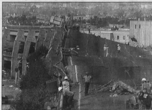
Workers check the damage to I-80 in Oakland Thursday. The freeway collapsed in Tuesday's massive earthquake.
