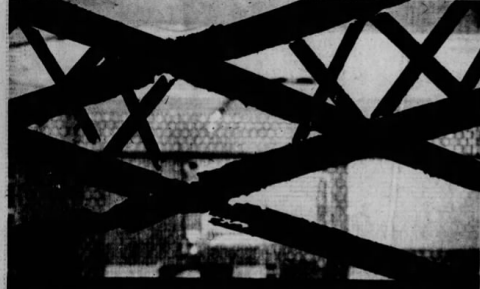
RICKETY BRIDGE: Rusted trusses beneath the automobile deck of the MacArthur Bridge. The bridge support stays the structure is several depths the deterioration. (Post-Dispatch Photo by Robert C. Mohr III)
