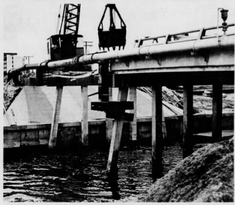
Workers continue construction on the final section of the Richard Beecher Bridge over Bass Inlet in Punta Gorda. The bridge tentatively is scheduled to open Wednesday.
