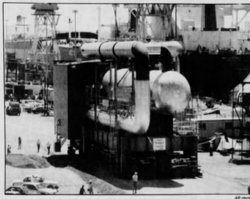
An 11-story tall modular building bound for the Alaskan oil fields is rolled toward a barge at Swan Island shipyard. The module, and others like it, are being shipped started this week.
